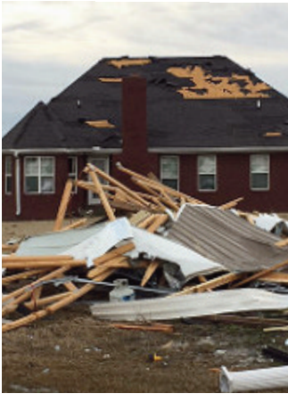
Mississippi County Extension agent Shawn Lancaster's home damaged and shop destroyed by a tornado Feb. 24, 2018.
