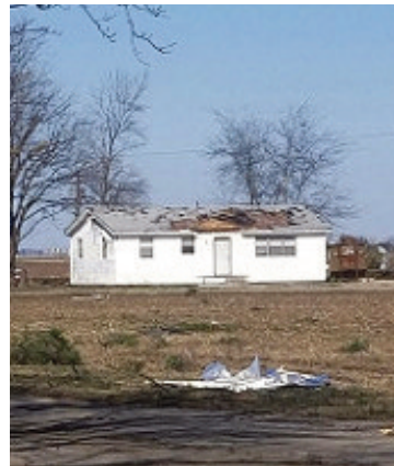
Roof of this residence at Northeast Research and Extension Center at Keiser was severely damaged during a tornado Feb. 24, 2018.
