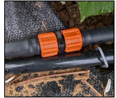
Figure 8: A coupling connecting two sections of drip tape after a leak was repaired.
