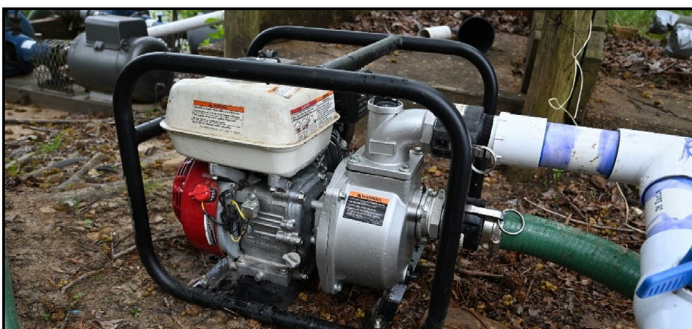
Figure 2: An irrigation pump.
