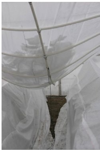
Image 3.5. The hoops of a caterpillar tunnel partly collapsed under the weight of a snow load.
