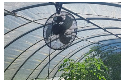
Image 4.26. A fan installed inside a high tunnel to help improve air flow throughout the structure.
